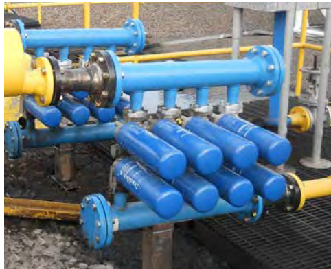
Single-pass Bulk Fuel Filtration System
